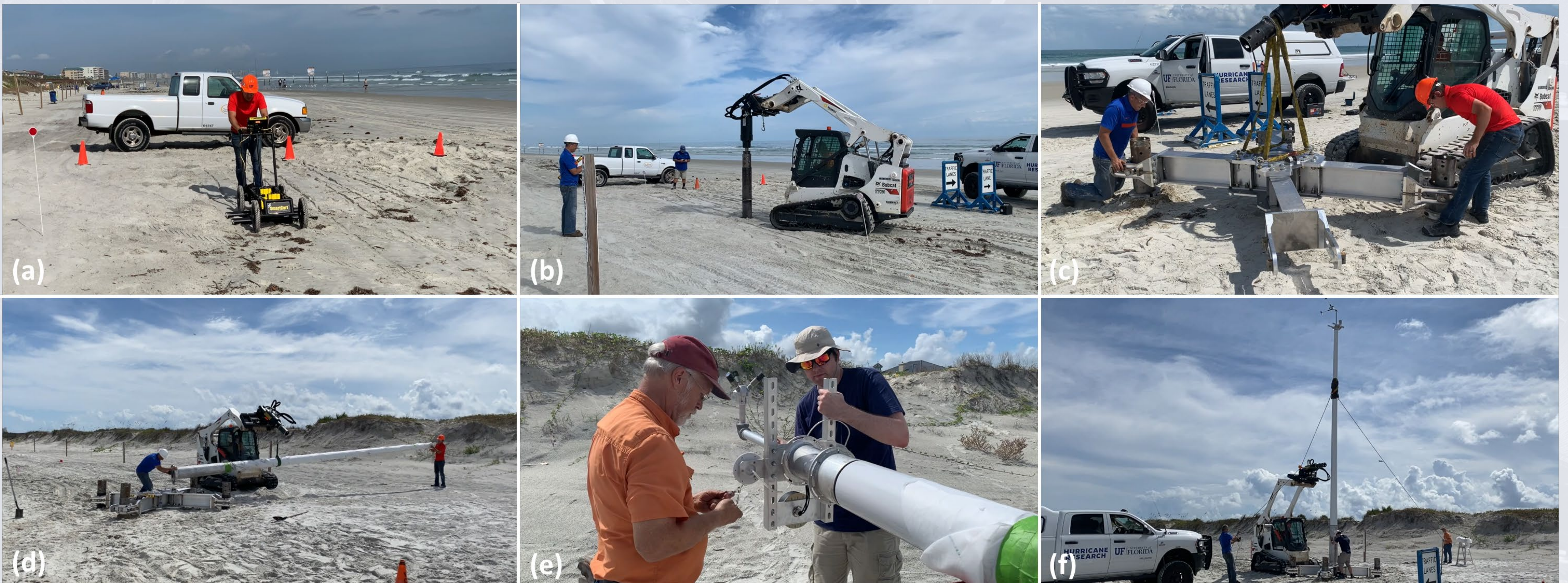
(a) GPR survey, (b) helical pile installation, (c) pier cap installation, (d) securing the 10-m mast, (e) inserting the instrumentation package, and (f) standing up the mast
